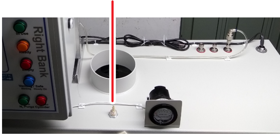
Exterior View From the Front - Acetylene Gas Cabinet
