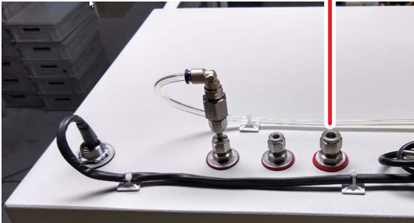
Exterior View From the Back - Acetylene Gas Cabinet
