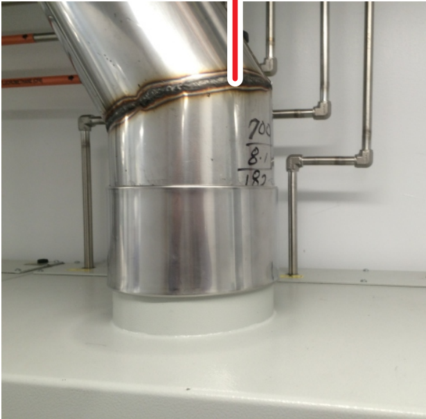
Typical Installation of Vent Conduit
