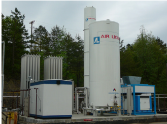
Used by permission from Air Liquide, the copyright owner
