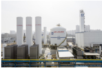
Used by permission from Air Liquide, the copyright owner
